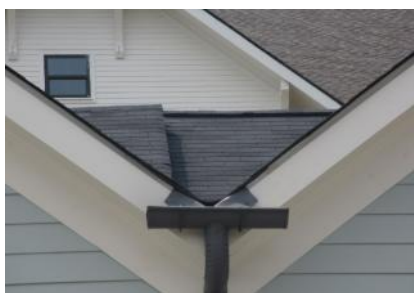
The weak roof slope along this valley is another potential concern.
