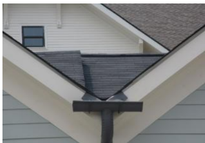
This gutter design is occasionally seen, but we aren't convinced of its adequacy in draining the roof.
