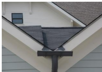
A very small section of gutter is expected to catch a concentrated flow of water and may not accommodate heavier storms.
