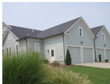
The weak roof slope along this valley should be monitored for future water penetration.
