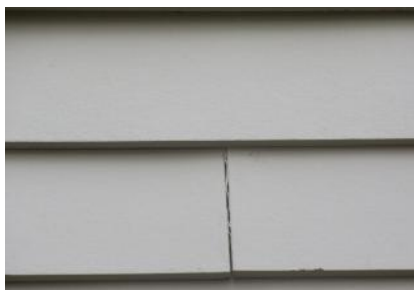
Some butt joints have opened up and should be caulked whenever buildings are painted next.
