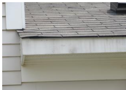
Eaves exhibiting water staining.
