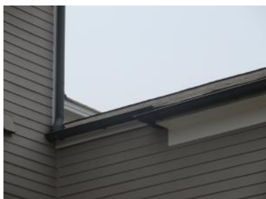
This is an unusual layout of gutter system. It may be or become problematic over time.
