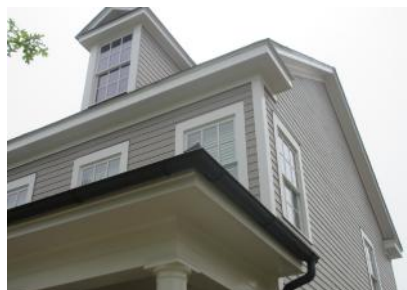
A substantial number of eaves lack gutters and downspouts which help to shed water away from the building.
