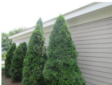
A substantial number of eaves lack gutters and downspouts which help to shed water away from the building.
