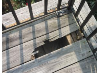
Side deck flooring needs to be replaced.
