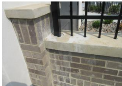
Holes should be filled to prevent water puddling and causing the fence to fail prematurely.
