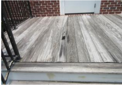
Side deck flooring needs to be replaced.
