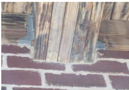
It's unusual to see brick installed up to joists. Board may wish to have this further investigated to determine if a problem exists. Located at clubhouse deck.
