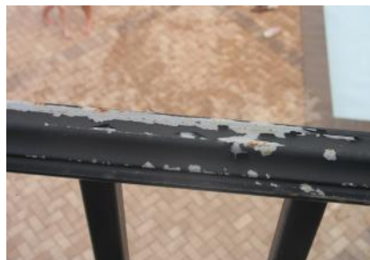
Club deck railing's finish has failed prematurely.
