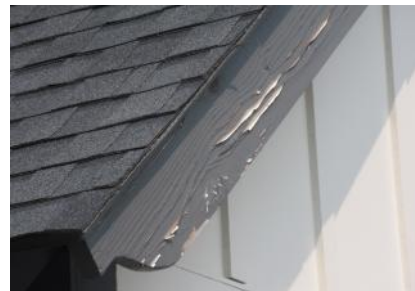
The paint is already failing along this rake even though it was just recently painted.
