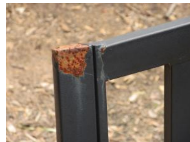
Protective coating has flaked off.
