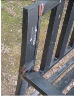
Protective coating has flaked off.
