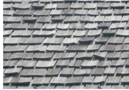
Cedar shakes are beginning to warp.
