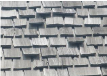
Some shakes have split. Most have shrunk leaving larger gaps between shingles.
