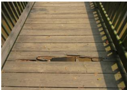
The bridge should have damaged floor boards replaced.
